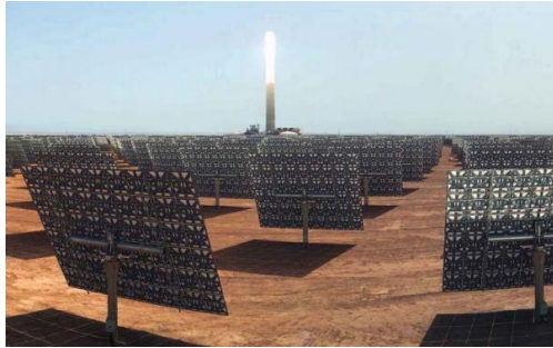
Figure 3. Heliostats installed at Noor III in Morocco; Source: Roadmap to Advance Heliostat Technologies for Concentrating Solar-Thermal Power, link to reference ?
